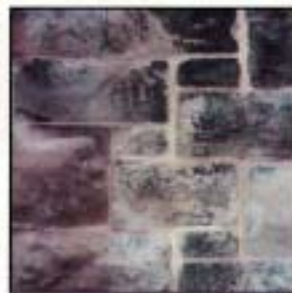
The erosion effects of rain and pollution weathering on soft sandstone.
