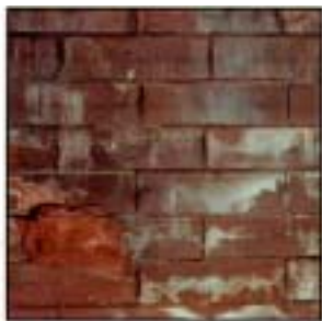
Old red brick with spalling decay due to moisture absorption and efflorescence.
