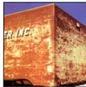
Due to excess moisture the white crystals of efflorescence salts deface the surface of a new brick wall and can cause future problems.
